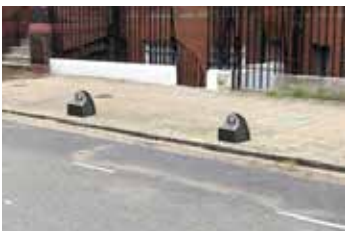
Figure 14: Connected Kerb Armadillo kerbside charge point
