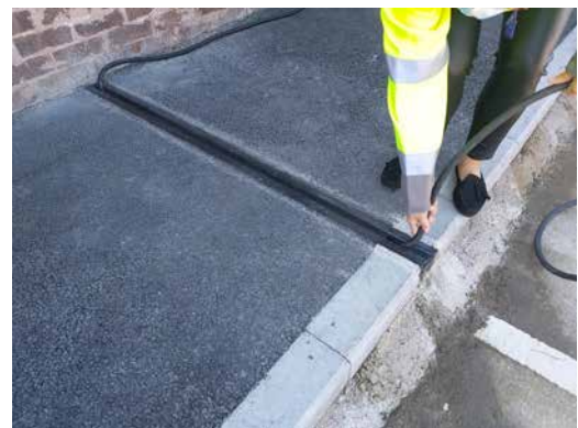
Figure 27: OxGul-e cable channel
