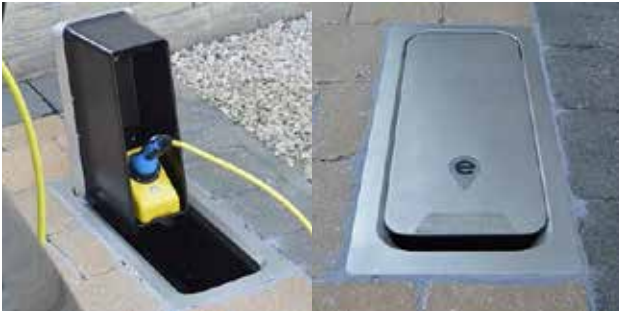
Figure 11: Street Plug underground charging solution
